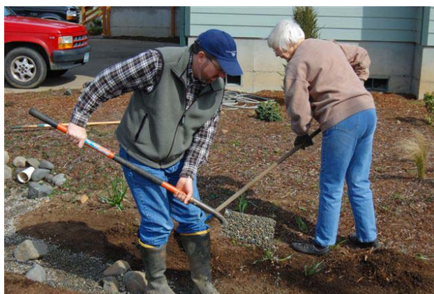
Rob Emanuel (L) and Pat Sears (R) installing part of the rain garden.
