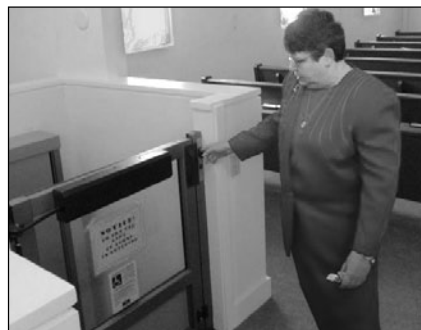
The Rev. Bobbi Neason presses the button to operate the new lift installed at First Presbyterian, Bandon.
